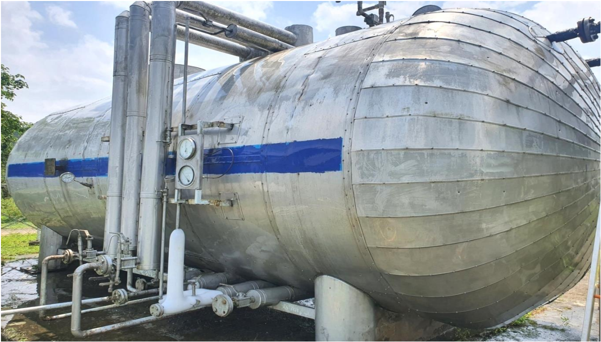
Fig. 30b.(Side-view) Liquid CO 2 storage tank (20 metric ton)
