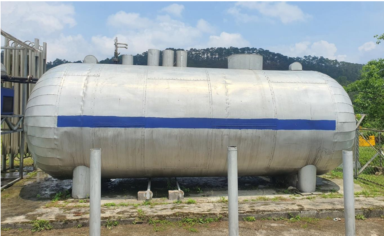
Fig. 30a.(Front view) Liquid CO 2 storage tank (20 metric ton capacity)
