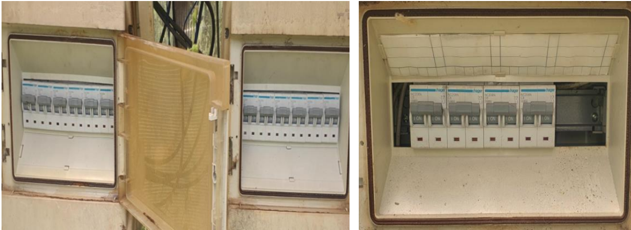
Fig. 22. (L) The MCBs of the IR heaters and (R) CO 2 solenoid valves
