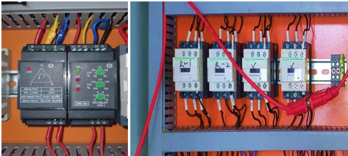
Fig. 15. (L) Single Phasing Preventer & Auto-Voltage Relay; (R) Contactors
