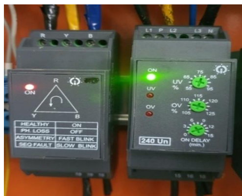
Fig. 19. Automatic relay (L) and Supply monitoring phase (R)
