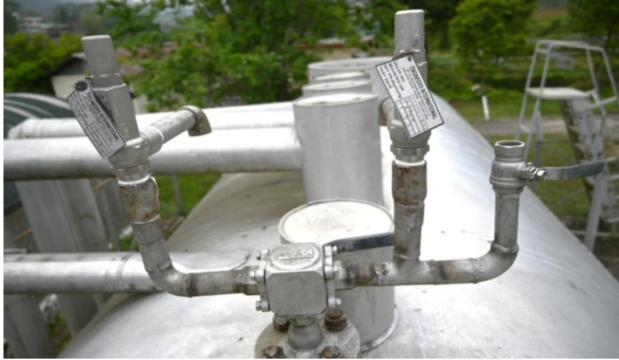
Fig. 32. Safety Relief Valves
