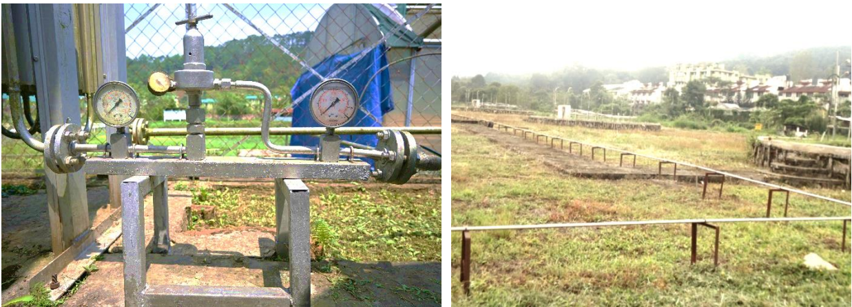
Fig. 31. Supply of CO 2 gas through Pipelines from tank to CTGC chambers and FATE Rings through safety pressure regulators and pressure gauges.
