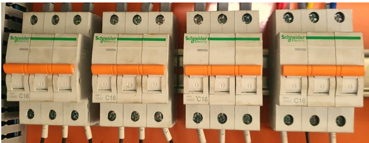
Fig. 21. Four MCBs for powering the four electrical contactors
