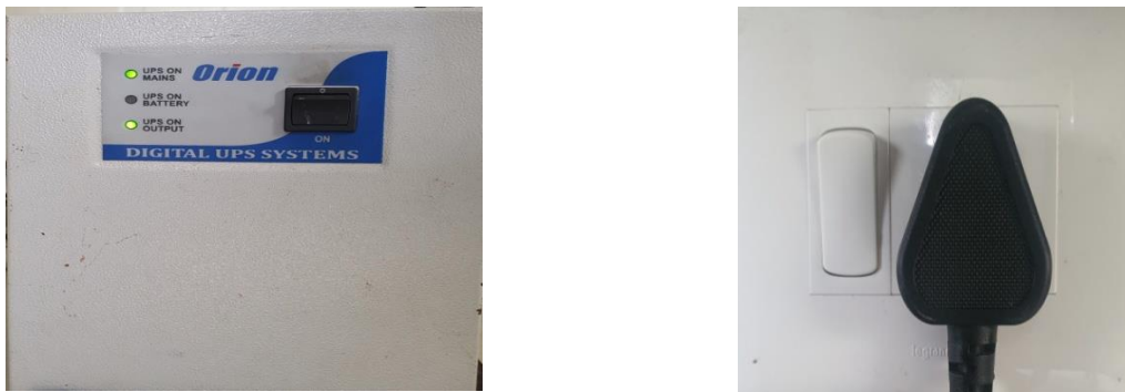
Fig. 20. UPS unit connected to a power source.
