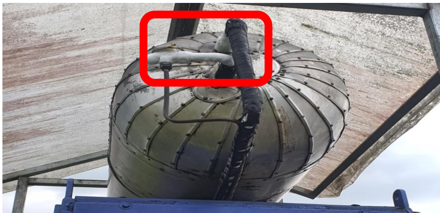
Fig. 37. Formation of ice (marked in red) in the Chiller machine
