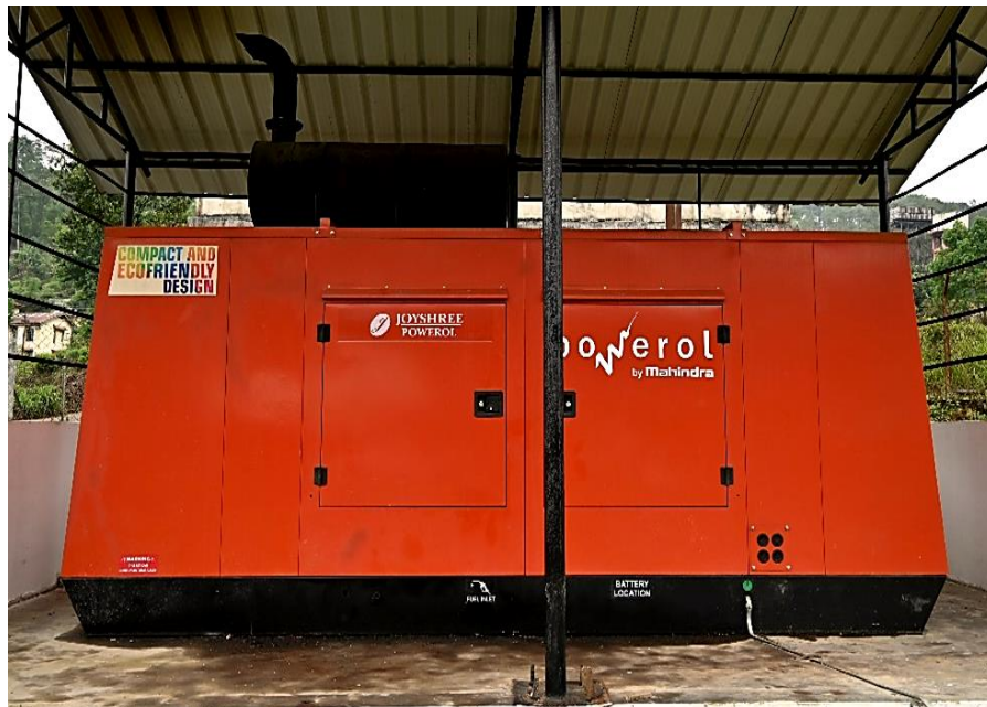
Fig. 38. The Diesel Generator use for power backup of FATE & Chiller
