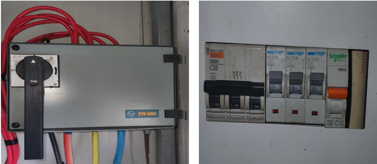
Fig. 18. (L)main line panel; (R)MCB for powering the control panel
